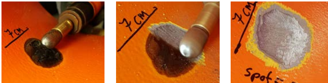
Corroded surface before and after treatment
